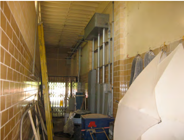
Electrical upgrades are installed unattractively, rendering this otherwise usable space good only for storage.
