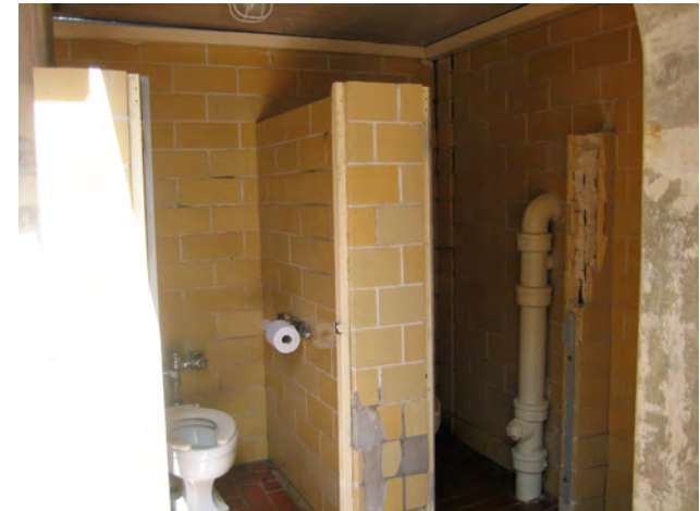
Aside from the deterioration, the preponderance of masonry toilet partitions gives the place a crowded feel. A rehabilitated Bathhouse should include more generous maneuvering clearances throughout.
