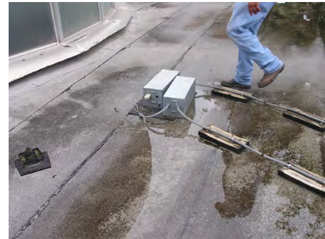
Most penetrations for roof top equipment electrical and refrigerant lines are voided and open.
