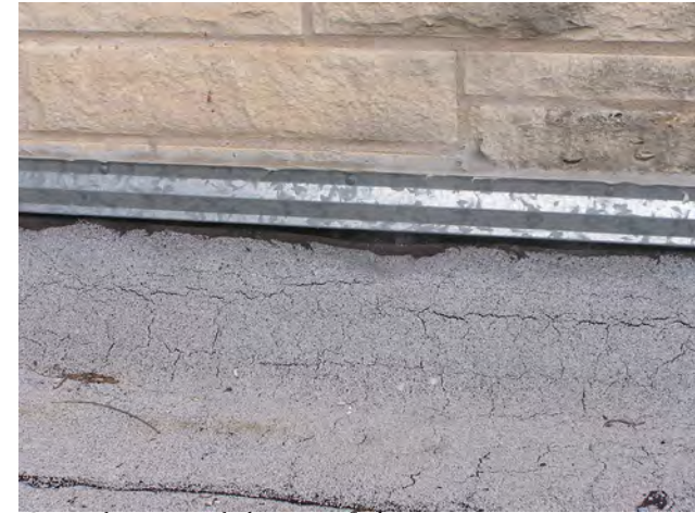
Certain locations include counter flashings at rise walls. Those metal flashings are voided in several locations.
