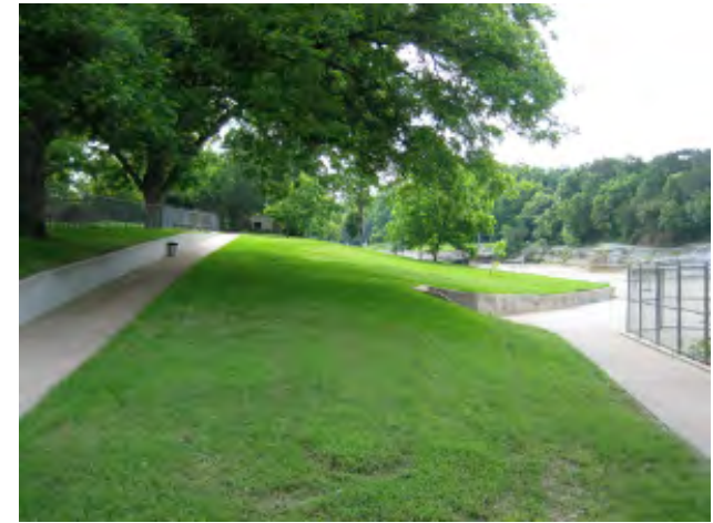
The slopes on the northside accessible route should be measured to verify that they meet the requirements of the ADA.
