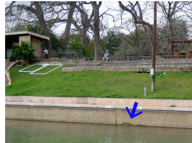
With water level down, gurgling leak in bypass tunnel is visible.
