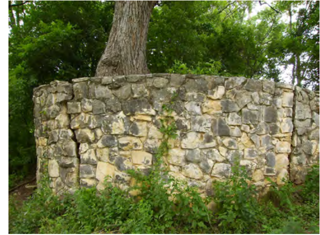
Repairing and stabilizing this crack will require the removal of the tree.
