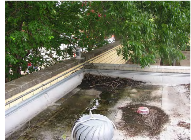
With a single area drain, and no overflow drain, a clog could lead to a catastrophic roof collapse.
